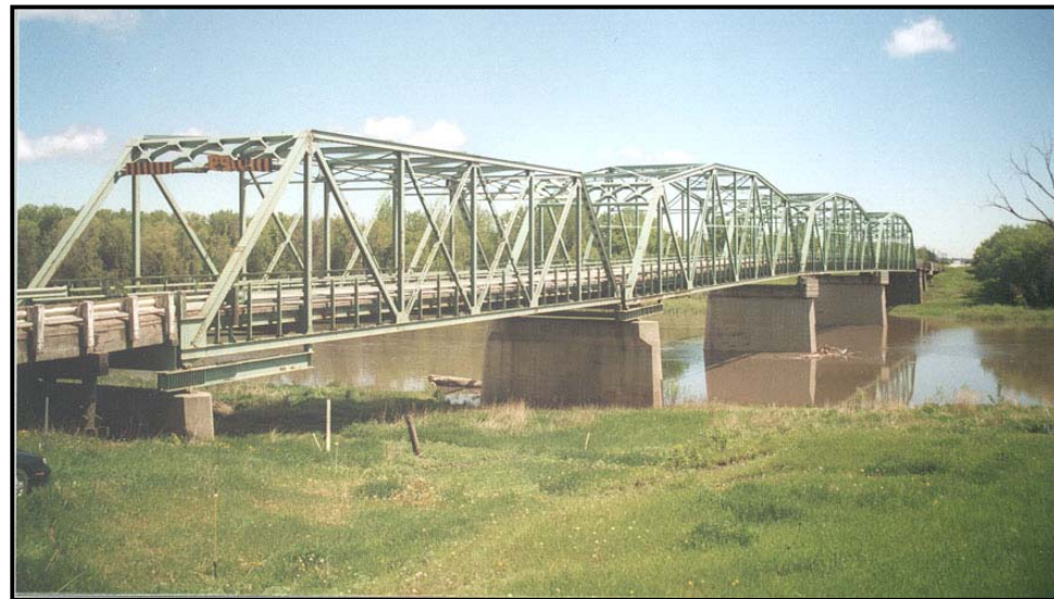
6.3.6 Above: Multi-arch steel truss bridge over the Red River at Letellier (Photo: Historic Resources Branch.)
