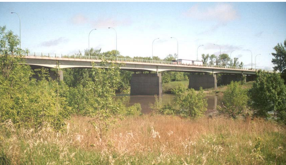
6.3.7 Above: Modern flat-deck steel-beam and concrete-pier bridge over the Red River at Morris (Photo: Historic Resources Branch.)
